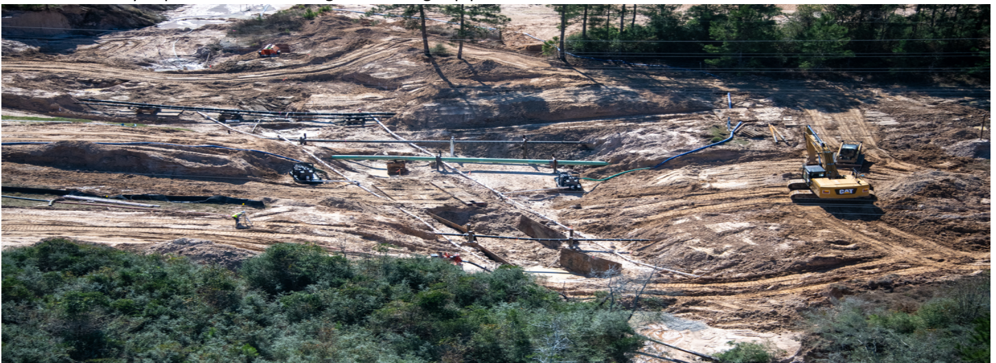
Workers attempt to shore up the pipelines to keep them from rupturing. We had a similar problem at the Triple PG mine where they exposed a Kinder Morgan natural gas pipeline.
