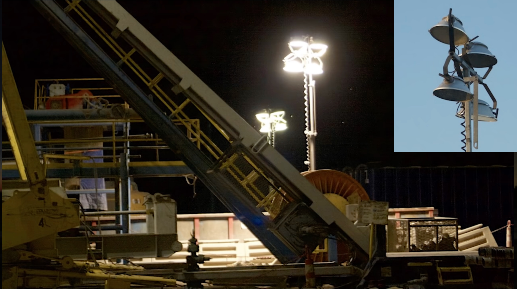
Sub-Optimal configuration. Stacked fixtures create glare off housing
